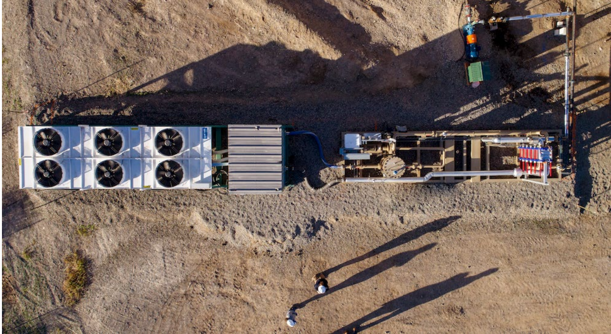
Figure 3. Drone imagery of an Electratherm AC800 ORC unit with six liquid loop radiator cooling fans on the left. Flexible hoses connect the ORC unit to the Sedna Sled Geothermal System on the right. For scale, note the people on the bottom of the image. Photo by Transitional Energy.
