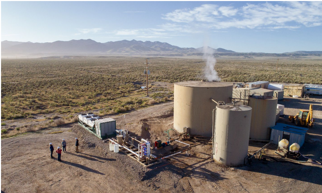
Image of Sedna Sled Geothermal System installed at the Blackburn Oilfield in Nevada.
