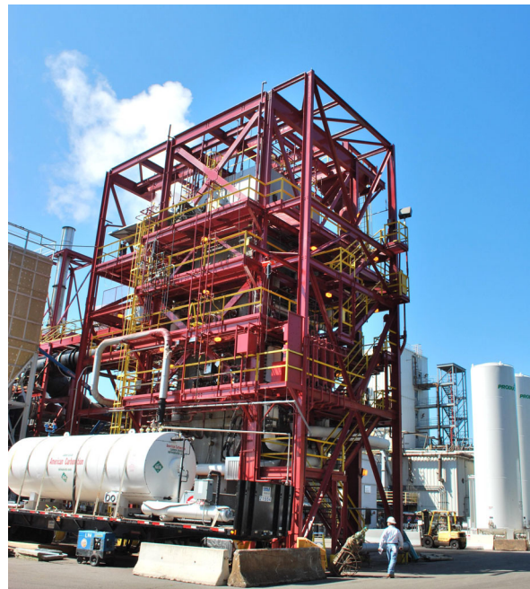
Figure 7 Boiler Simulation Facility
