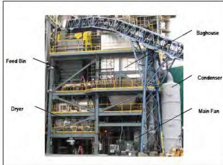
Figure 3-5 PSDF Fluid Bed Dryer System
