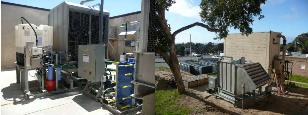
Figure 4. ESTCP demonstration hygroscopic cooling systems, Fort Irwin, California (left) and Seaside, California (right). The Fort Irwin demonstration began July 2018 and Seaside started March 2019. Both demonstrations will run through the 2019 cooling season.
