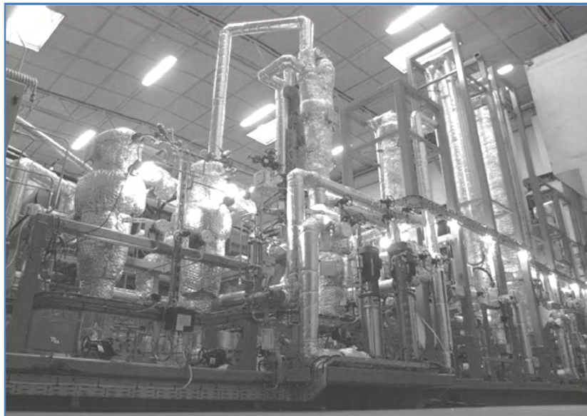
Figure 1 -- The Test Rig to be used (as installed at Consol Energy Research Center)
