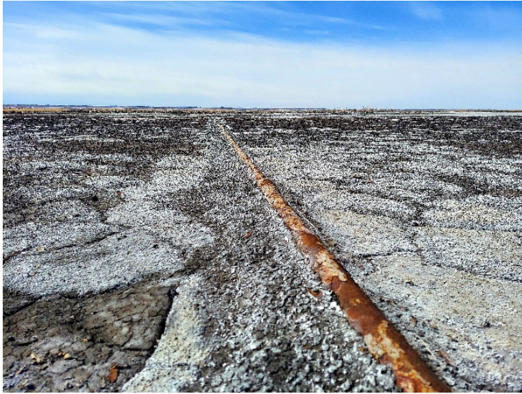
Beaver Lake exposed pipeline and salt contamination
