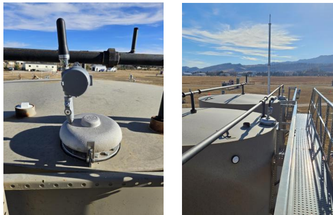
Figure 1: Typical Well Site Storage Tank with Device Installed
