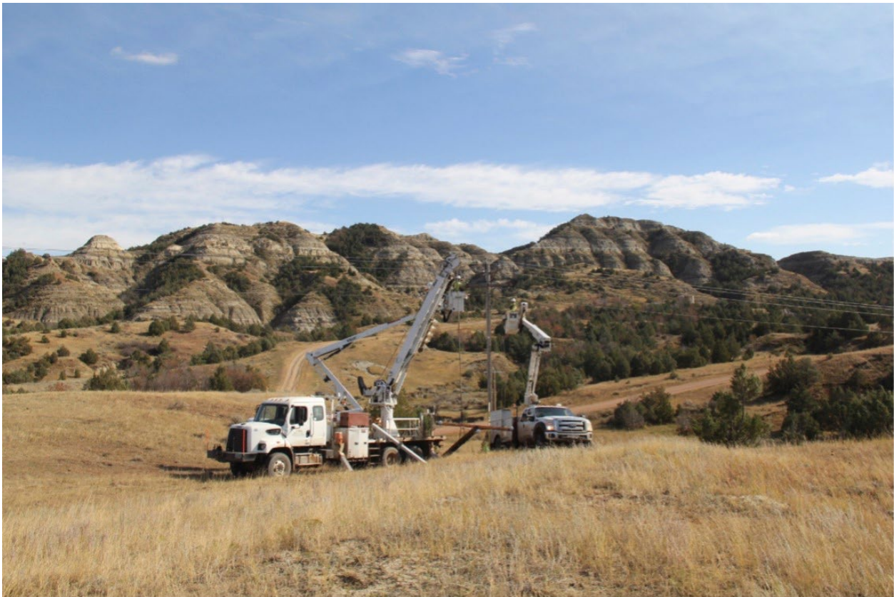
Photo courtesy Andrew Spratta – McKenzie Electric Cooperative
