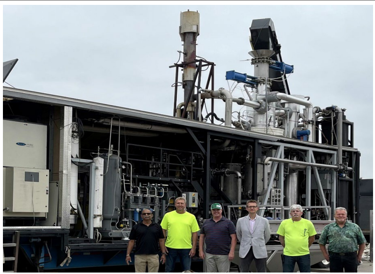
Figure 4. Five ton/day truck mounted Sandwich gasifier currently located at Tri-Steel Manufacturing.
