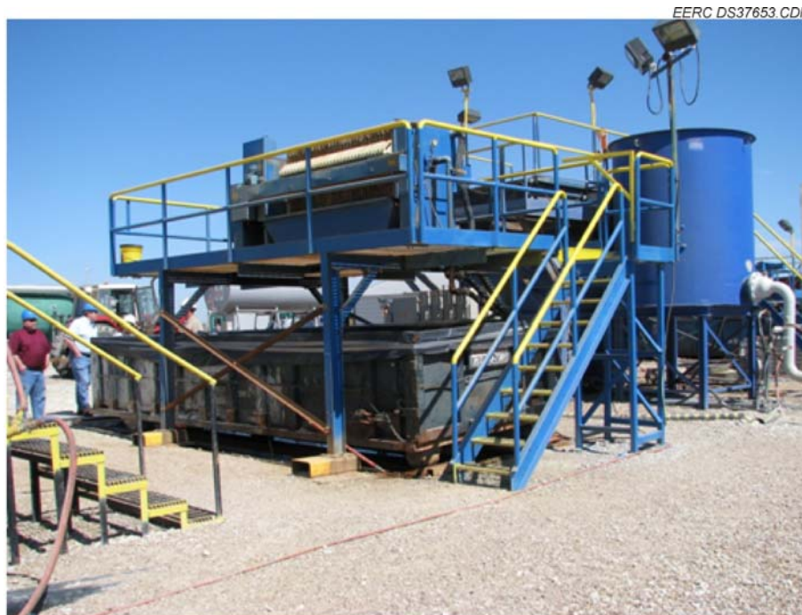
Figure 15. Pretreatment system consisting of coagulation/flocculation, settling, and filter press.
