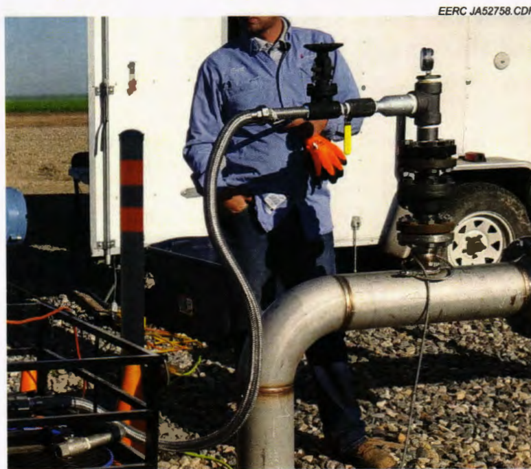
Figure 5. Metering skid connection to the gathering pipeline.
