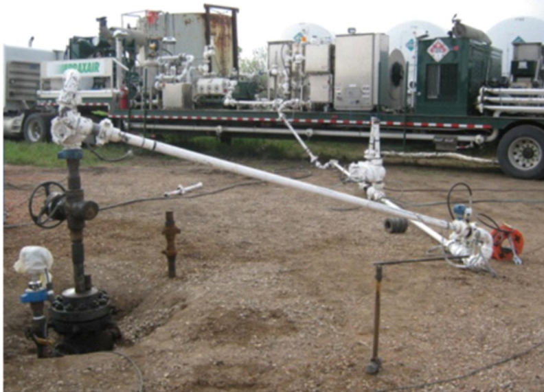
Figure 4-7. Pumping unit and pipe and valve system used to inject CO 2 into the E. Goetz #1 well.
