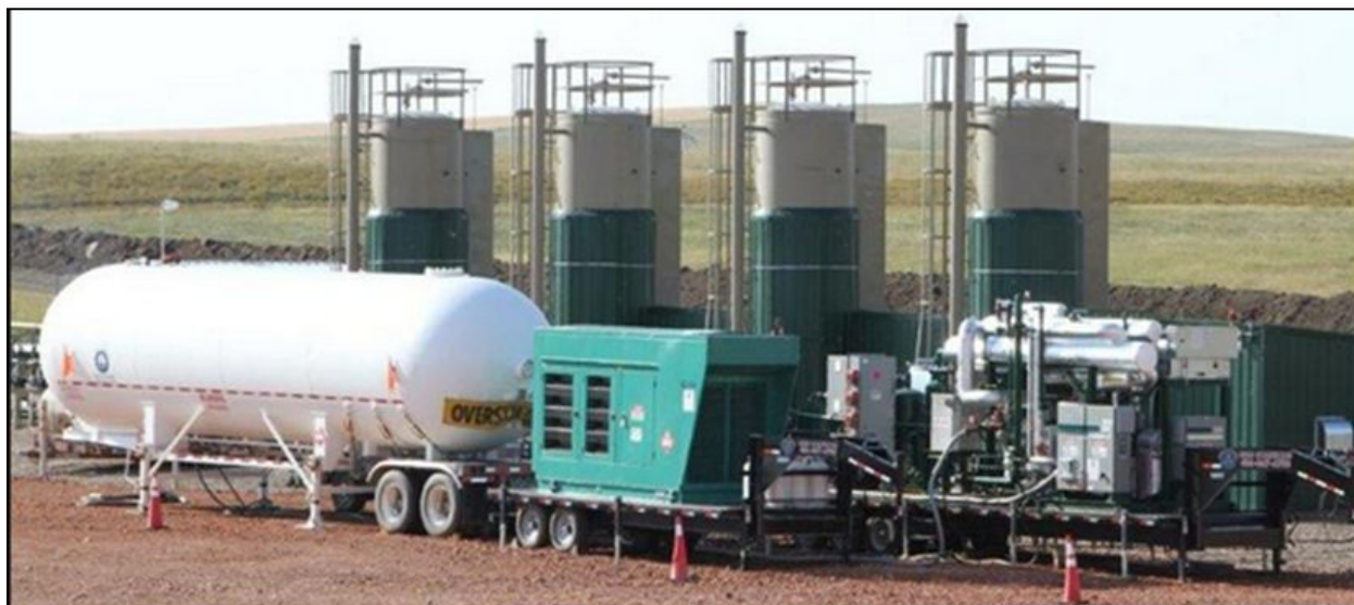
Typical NGL processing facility at a well site.
