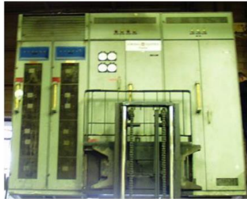
Thyristor Controls for Mud Pump
