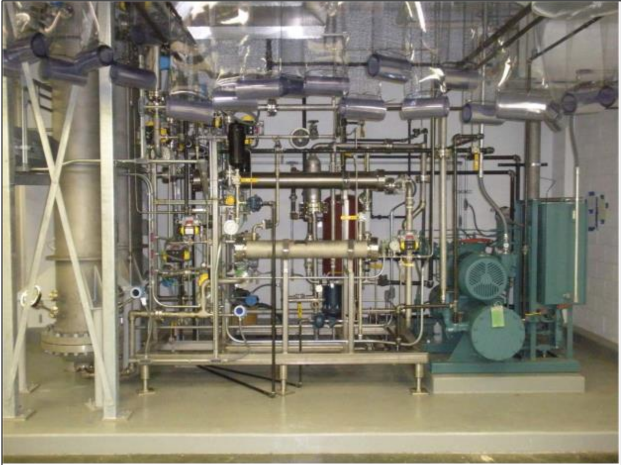
Figure 20. Pilot plant AFEX 3 system located at MBI
