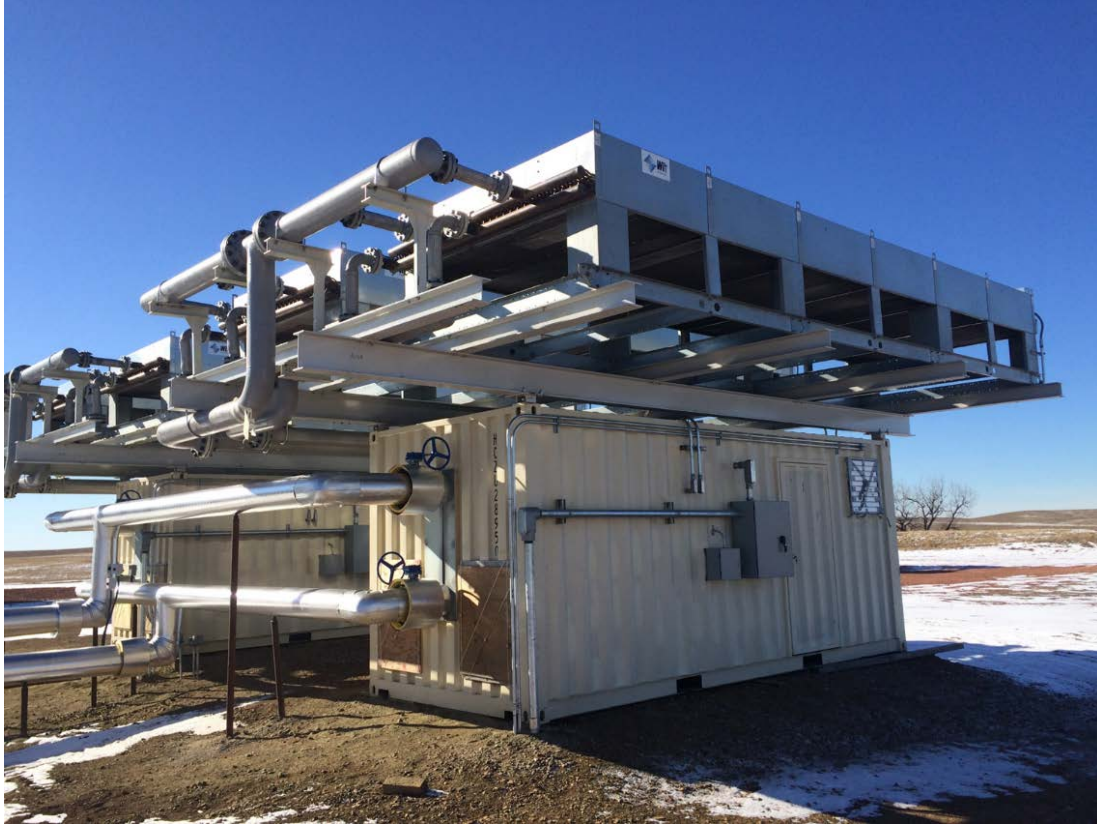
Figure 1.5 ORC units as installed at the Davis Water Injection site.
