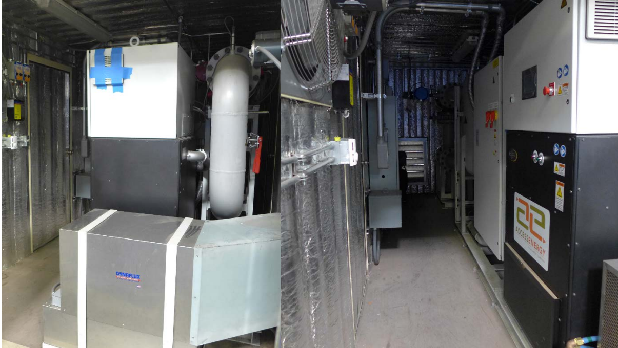
Figure 1.6. Inside of shipping container showing ORC system and control unit
