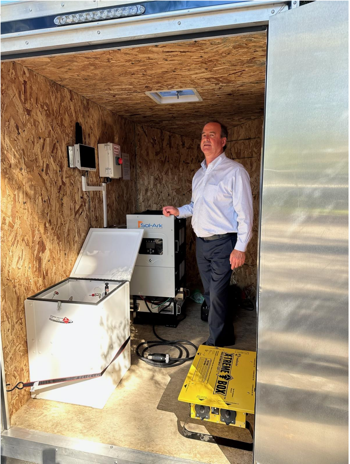
Figure 3. Spectator at CARB Demonstration, examining BWR Innovations zero-emissions generator
