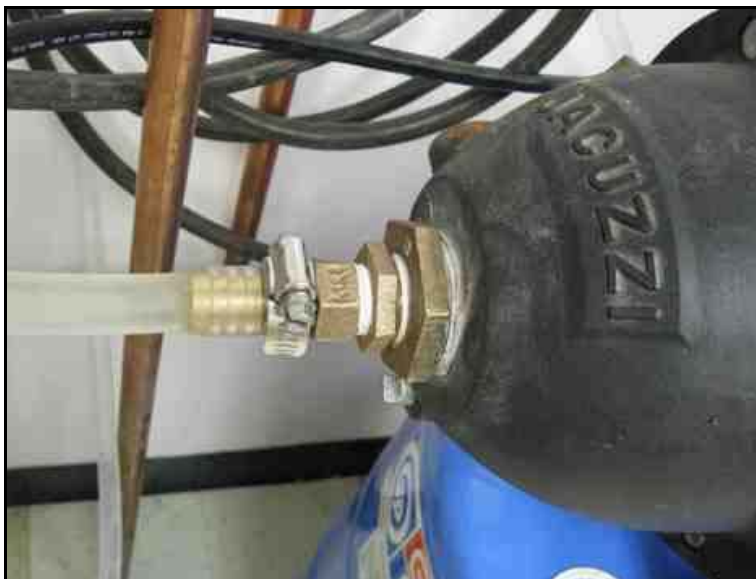
Fig. A4-2. Bladder air pressure arrangement for pressurized water supply to equipment
