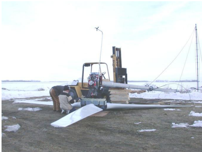
Installing the blades on Proto-1 This was a fixed blade – downwind machine.
